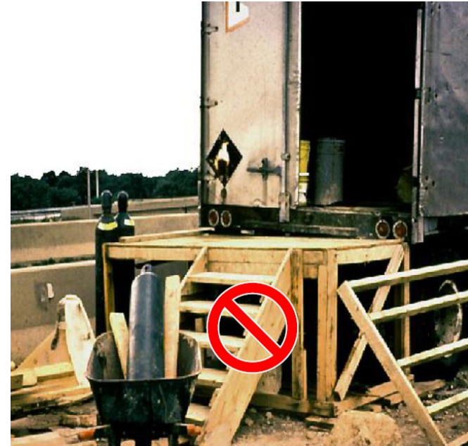
The stairway to this platform has more than 4 risers and is not guarded.
